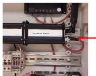
Figure 8e: Power Connected
