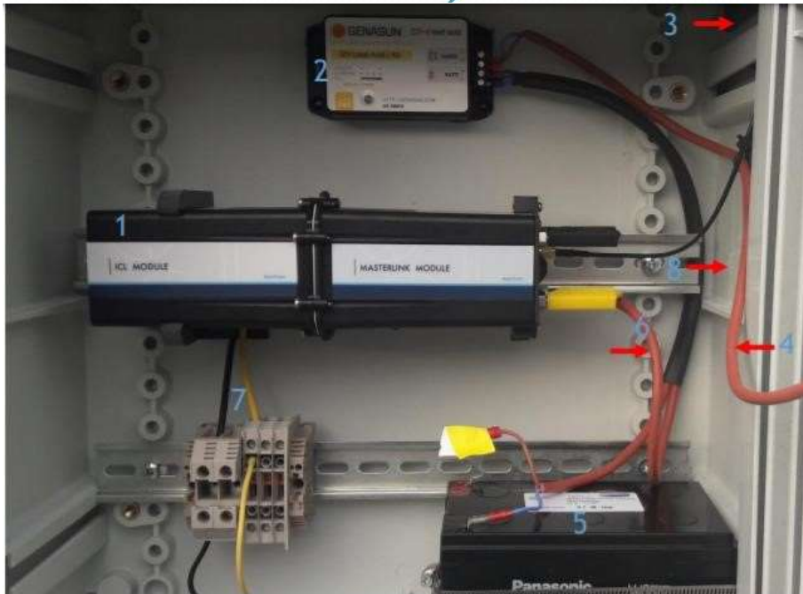
Figure 8ai: Interior of Single ICL Solar Junction Box as
